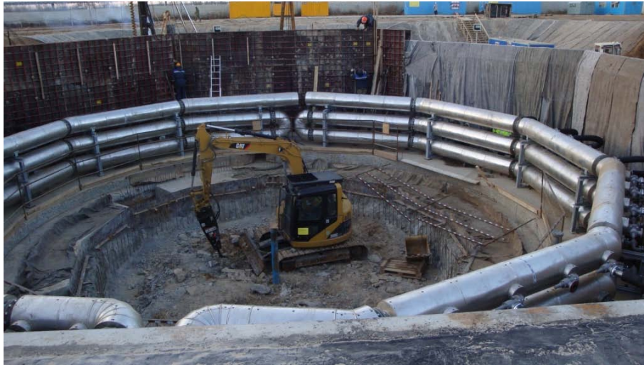
Skip shaft and cooling system pipes
